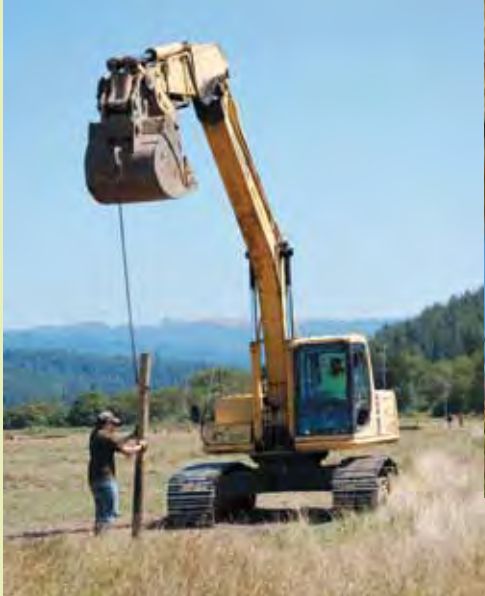
NRLT project manager Ryan Wells and Greg Turner from Hooven & Co. pull posts from the old fence line.
