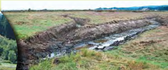
Two slough branches meet near Wood Creek. In all, more than 3,700 feet of slough channels were constructed on the project site.
