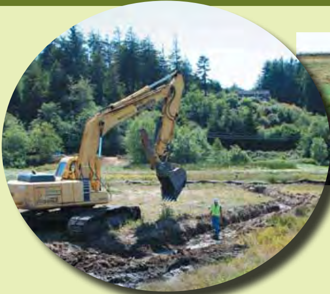
Another channel is nearly finished. This phase of the project will be completed when the existing tide gate at the mouth of Wood Creek is removed in October.
