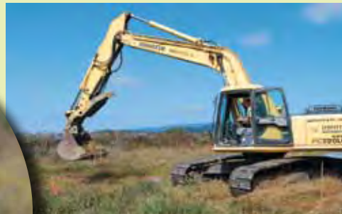
Salvaging Lyngbye sedge ( Carex lyngbyei ), a sensitive wetland plant species, from the project footprint prior to excavation. The salvaged plants will be potted and used for re-vegetation scheduled for next spring.
