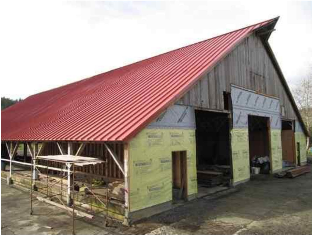
A new red roof on the barn can be seen by passersby on Myrtle Avenue near Freshwater Road.
